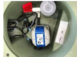
Inside the Control Turret
