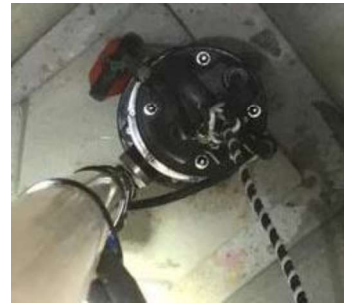
Pump Station / Irrigation Chamber
