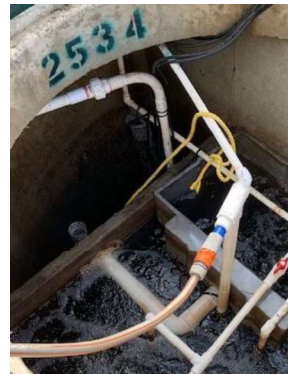
Flushing sludge return pipe
